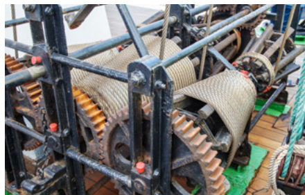
Deck & Cargo Handling Machinery
